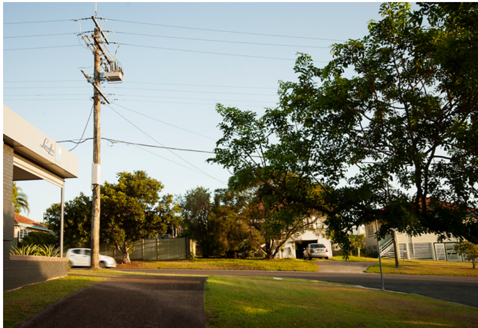
NOJA Power OSM Recloser Installation.
